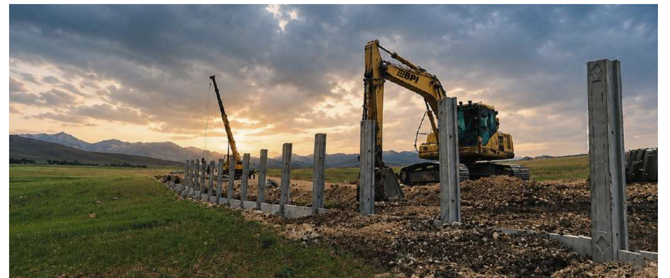
• Paband Zanja Solar Power Plant Project
